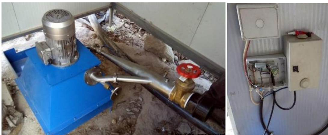
Figure 17. Pilot plant in the mine reservoir in Portugal.
