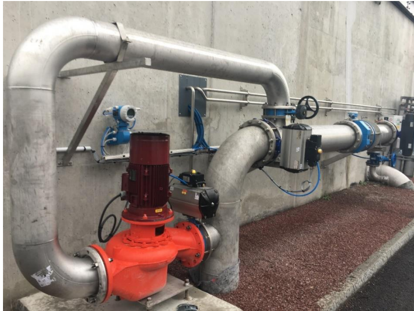
Figure 6. PAT installed on a bypass in the pilot plant in the drinking water sector in France.
