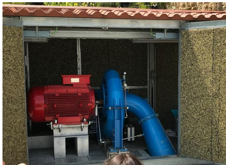
A turbine in a water supply network in Asturias (Spain)
