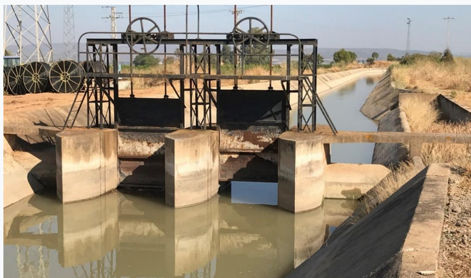
A sluice gate in an irrigation canal
